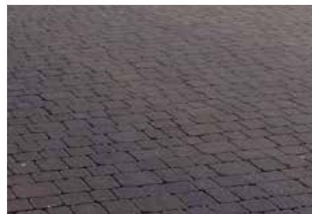
Highway - Tumbled concrete paviours
