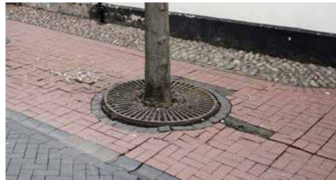
Paving effected by root heave (above)
